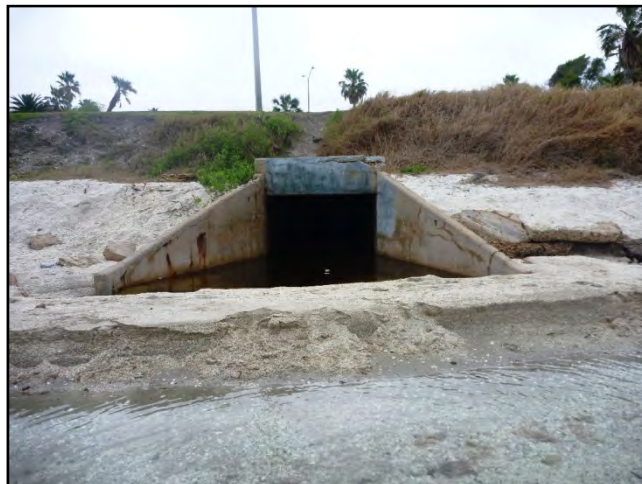
Fig. 2.21. Views of Poenisch Park with A) sandy and concrete rubble shoreline looking northwest towards downtown Corpus Christi, B) shoreline looking southeast with typical bank profile, and C) storm water outfall with stagnant pool of water.
