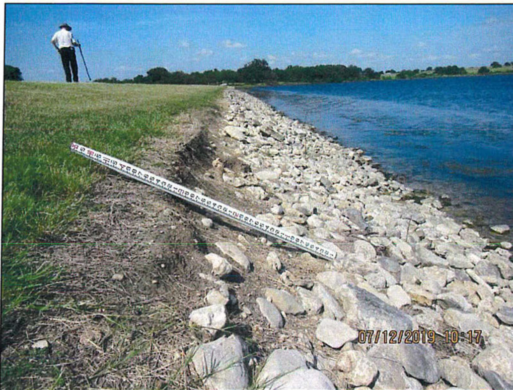
Photo 7 – Upstream slope. Looking right. Note displaced riprap and benching erosion.
