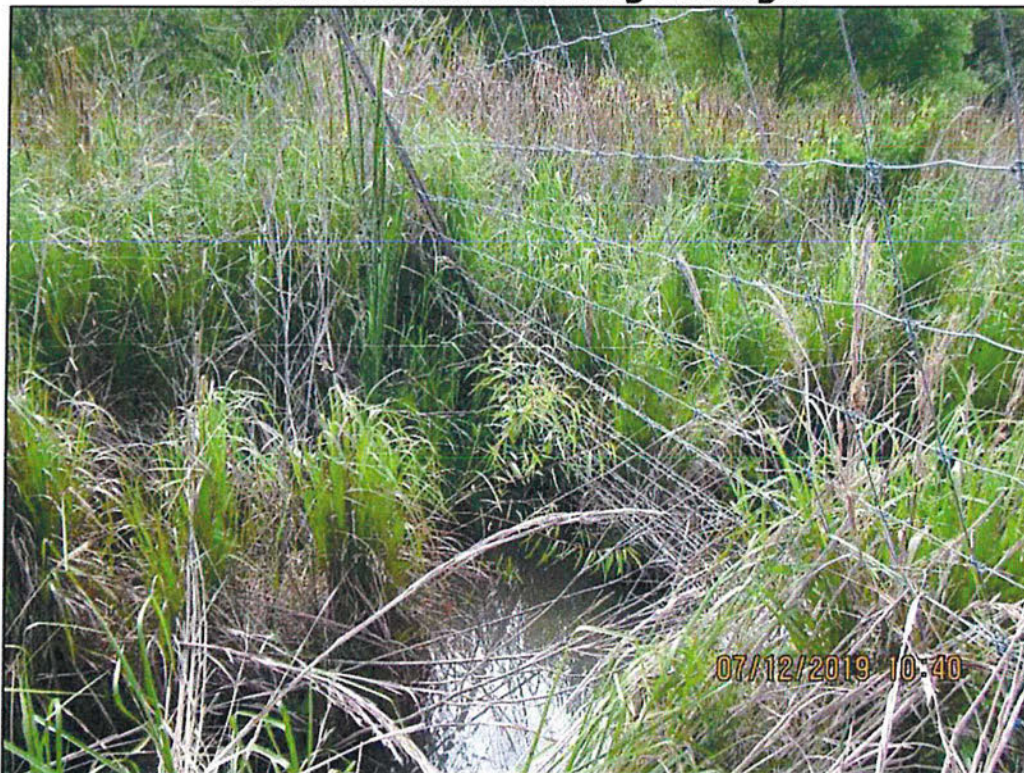
Photo 16 – Downstream toe. Mid dam. Note seepage.
