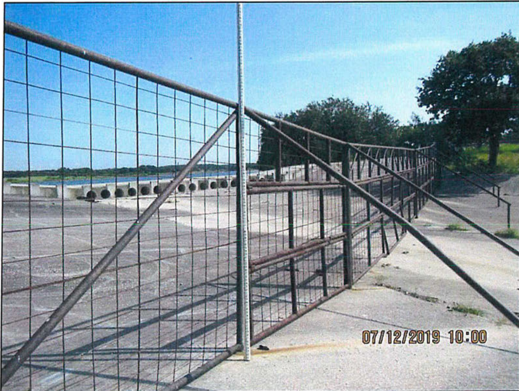
Photo 23 – Service spillway. At right side looking upstream. 8-foot fence with flap gate sections. Note corrosion.
