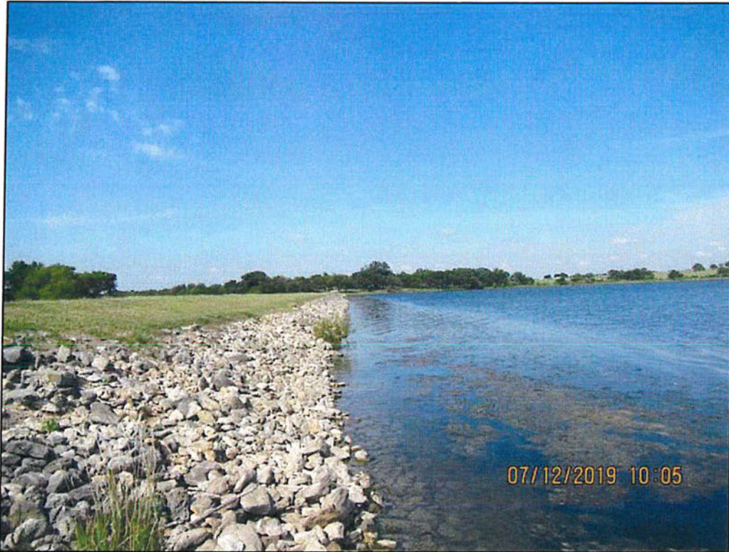
Photo 5 – Upstream slope. At service spillway. Looking right. Note minor vegetation in riprap.
