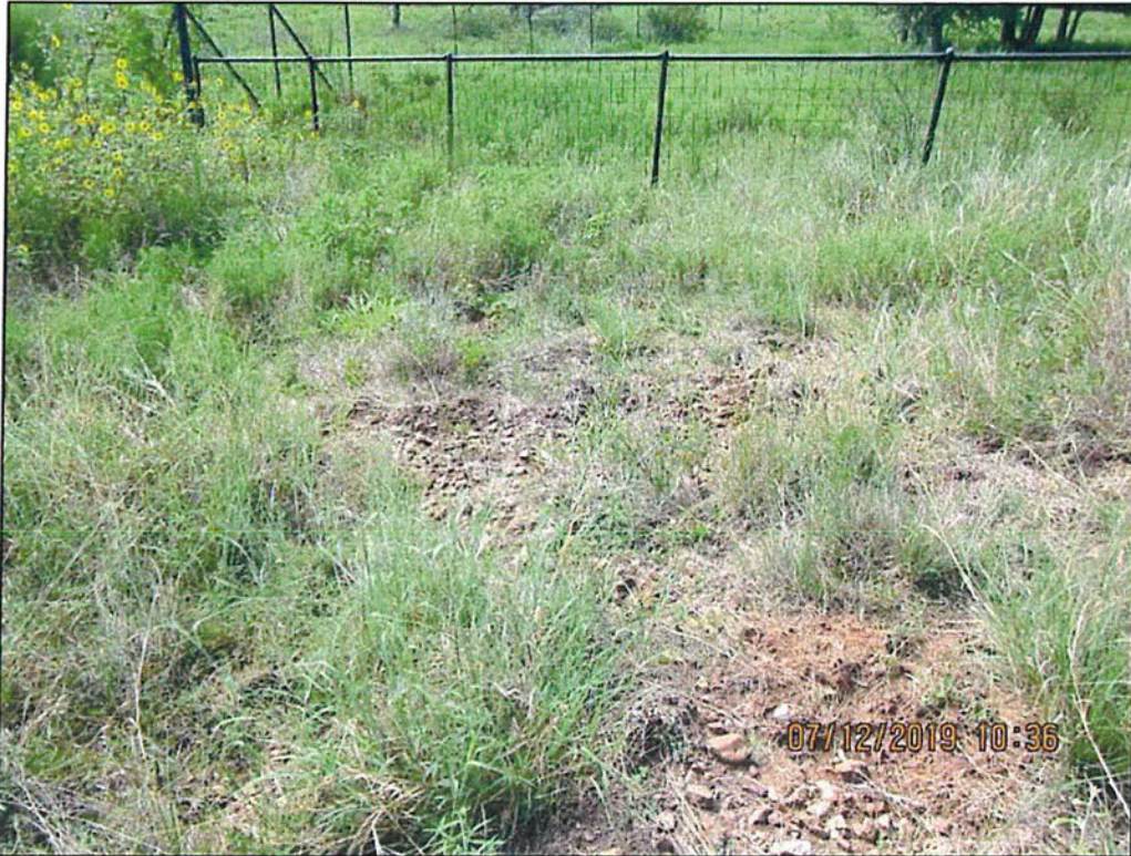
Photo 15 – Downstream slope toe. Near right end. Looking downstream. Note hog damage.
