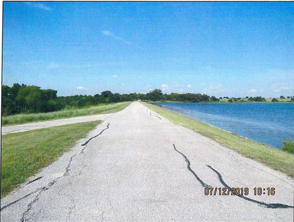
Photo 1 – Crest. At service spillway. Looking right. Note cracking in asphalt concrete.
