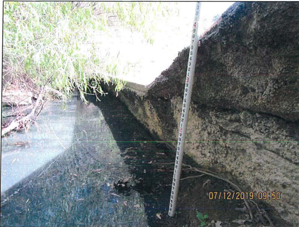
Photo 25 – Service spillway. At downstream end. Note undermining erosion.
