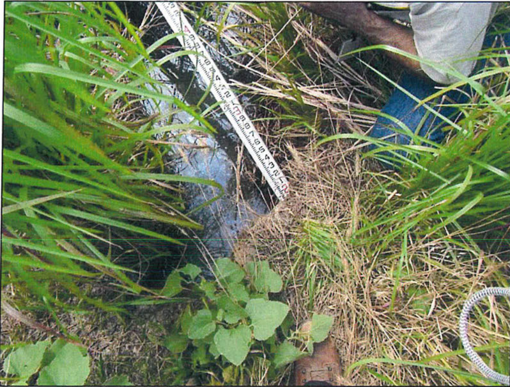
Photo 17 – Downstream toe. Seepage. Note animal activity.
