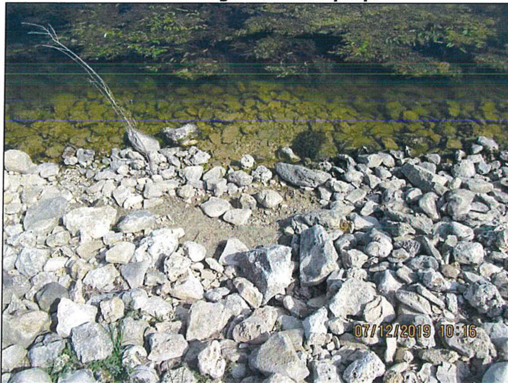
Photo 6 – Upstream slope. Displaced riprap and exposed embankment.
