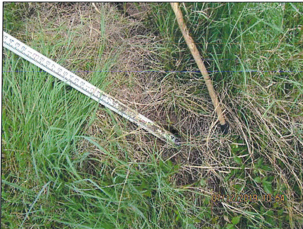
Photo 18 – Downstream slope. Typical animal burrow.
