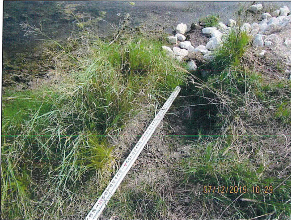
Photo 9 – Upstream slope. At right end of riprap section. Note erosion.
