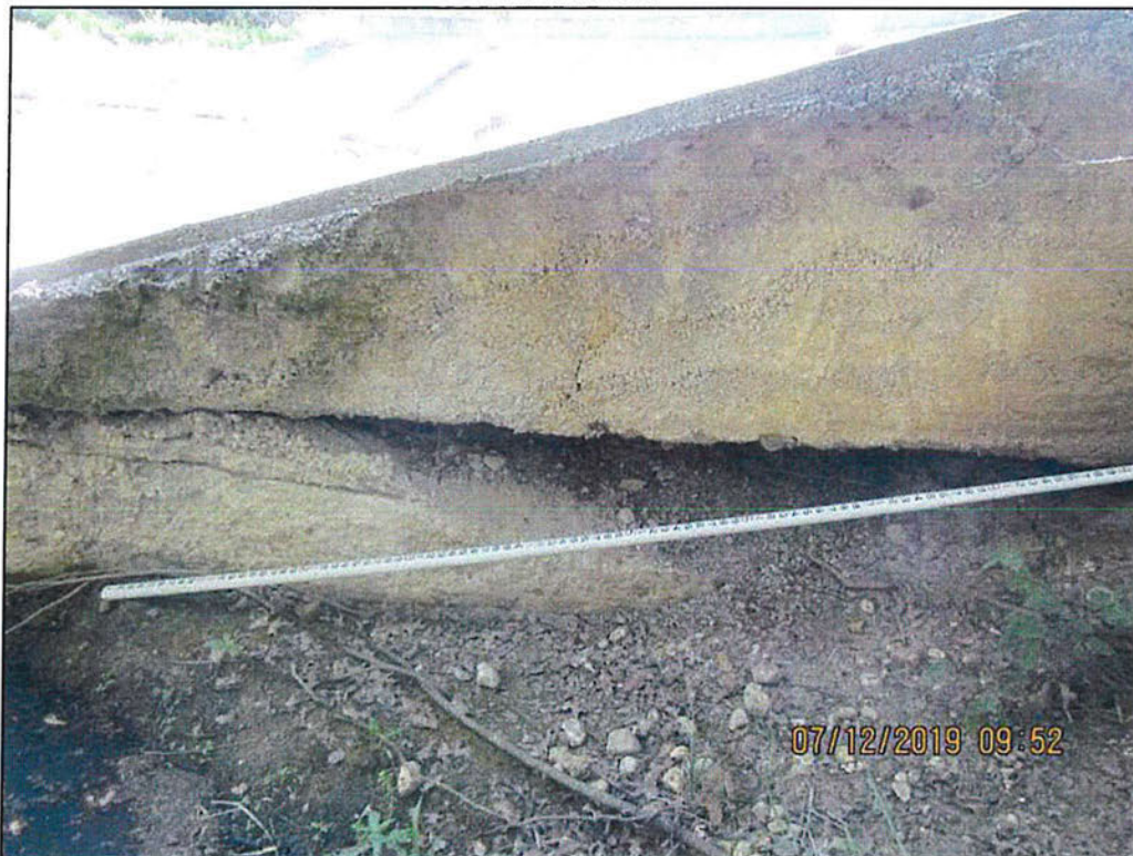
Photo 26 – Service spillway. At downstream end. Note undermining erosion.
