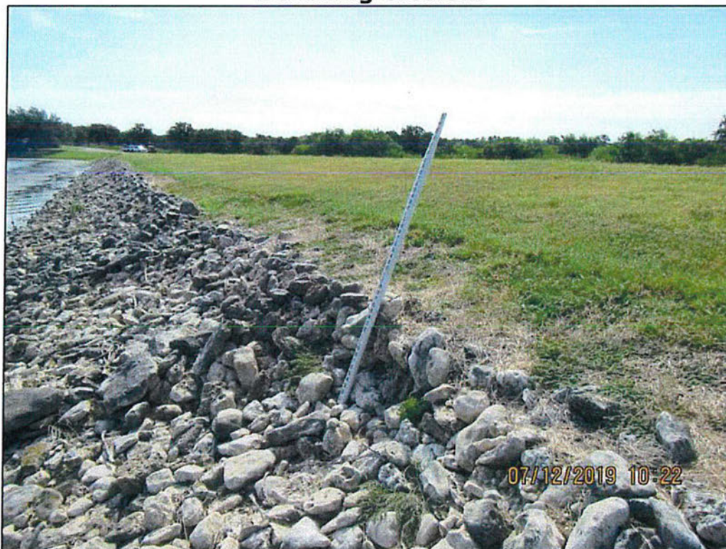
Photo 8 – Upstream slope. Mid embankment. Looking left. Note displaced riprap and benching.
