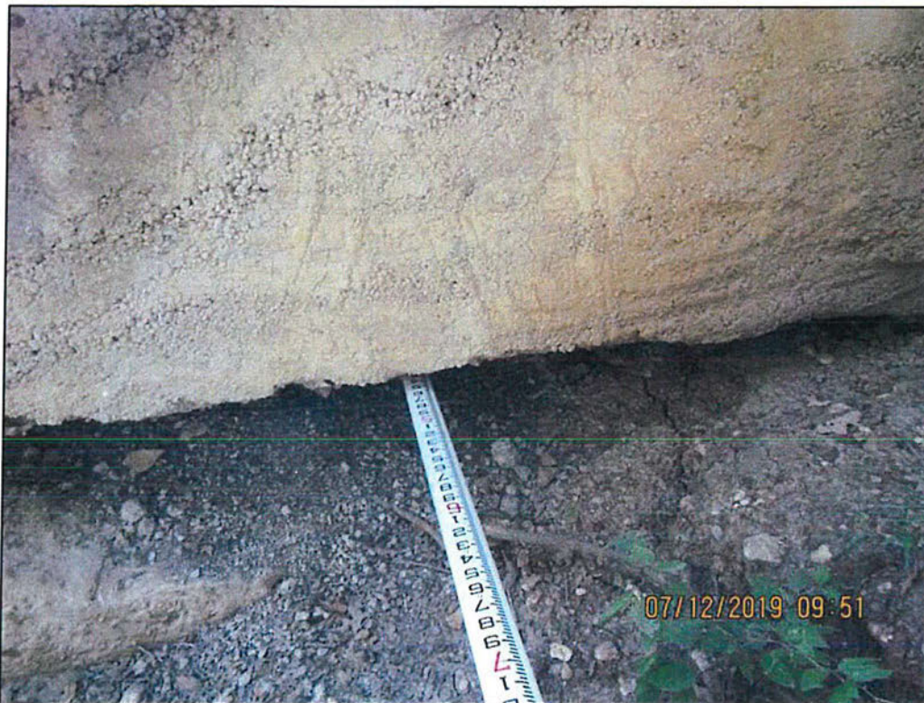
Photo 27 – Service spillway. At downstream end. Undermining erosion probed to 4.5 feet.
