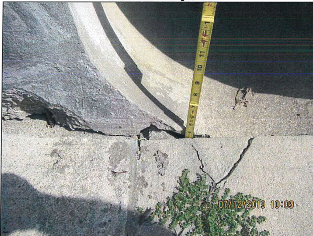
Photo 22 – Service spillway. Culvert pipe outlet at right end. Note spalling, cracks, voids, open joints, exposed reinforcing steel.
