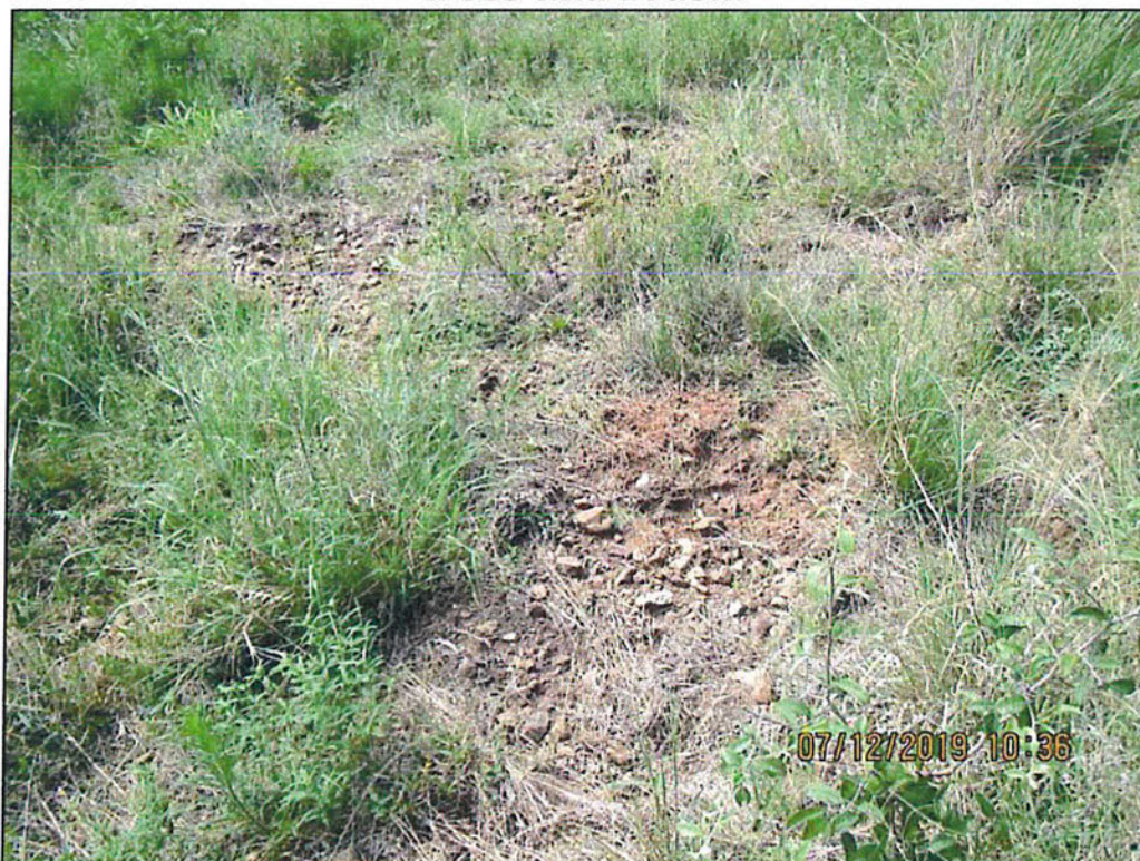
Photo 14 – Downstream slope. Near right end. Looking upstream and to right. Note hog damage.
