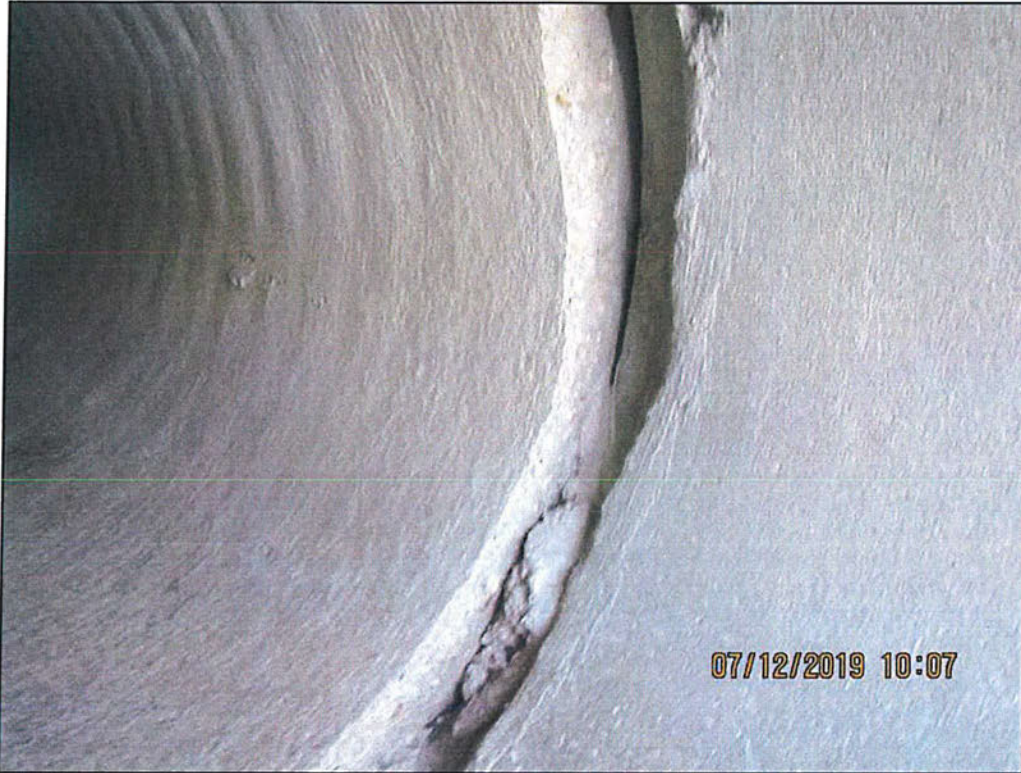
Photo 21 – Service spillway. Upstream side. Note typical gaps in construction joint.
