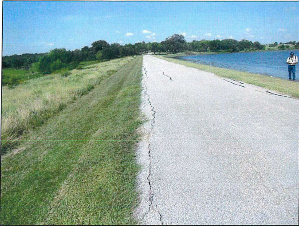
Photo 3 – Crest. Looking right. Note asphalt concrete cracking.
