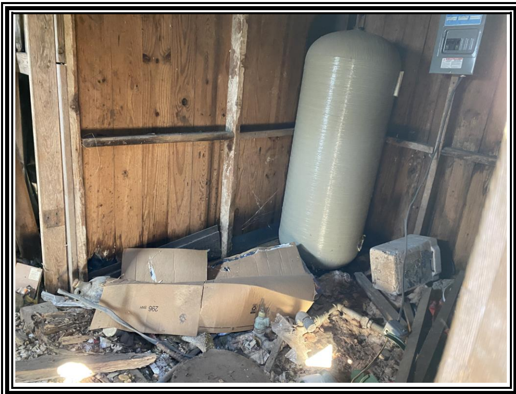
2. View of man made water well feature S-2, located south of the residence in the central portion of the tract.
