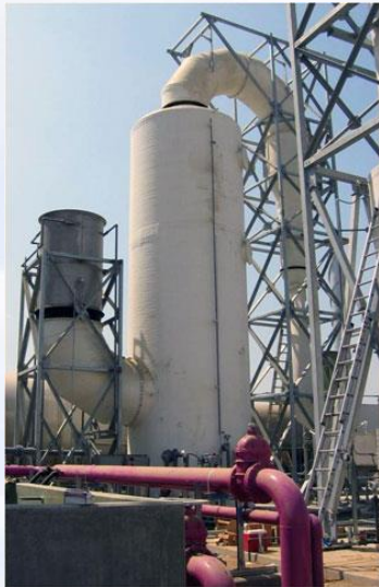
SO 2 scrubbers installed at power plant in Texas
